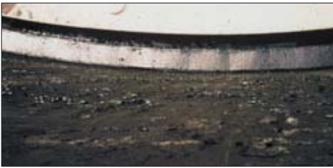
Tank wall without ...
